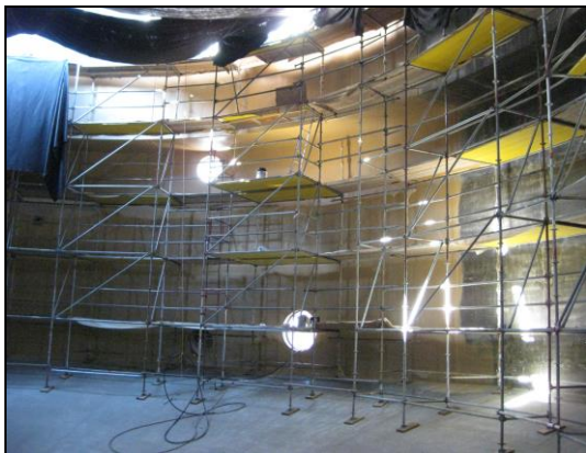
A single 60-mil coat of No. 210S was applied to all surfaces
