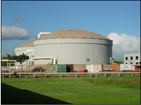
Exterior View of new Anaerobic Digesters
