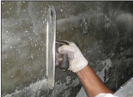
Following sandblasting operation, all concrete surfaces were skim-coated with No. 209 to fill bugholes and voids
