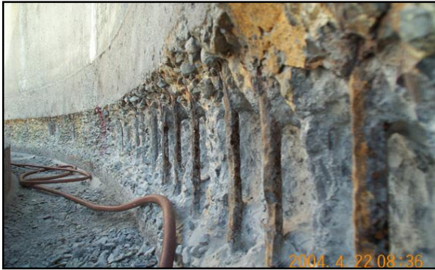
Eroded and corroded trough wall following hydro-blast prior to rehabilitation.
