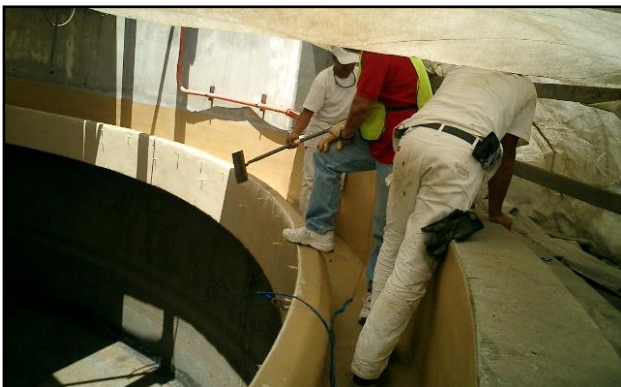
Rehabilitated trough protected with SewerGard 210T and 210G top coat to ease cleaning and maintenance.
